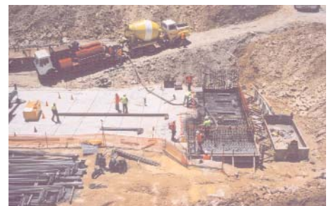
Recent scenes at the first structural concrete pour to the base of the Main Tower Lift Core
